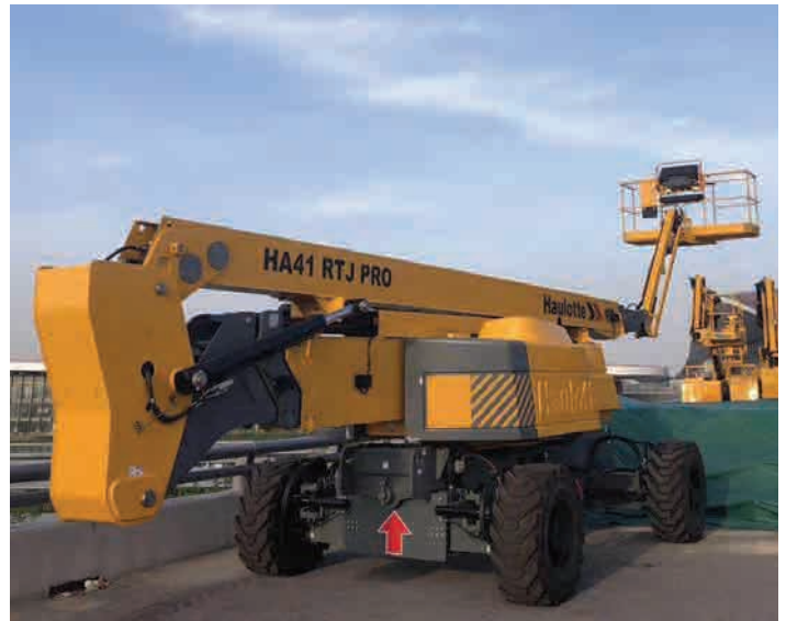
ALL IMAGES: Haulotte has delivered 16 machines for the construction of Beijing Daxing International Airport, including six articulating booms (two of which are electric models), two lightweight self-propelled booms, two vertical masts and six scissor lifts.
